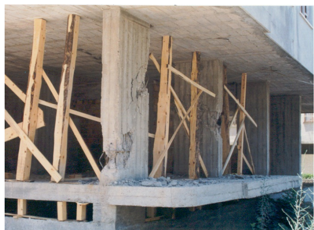
Fig. 7. Shear failure mechanism
