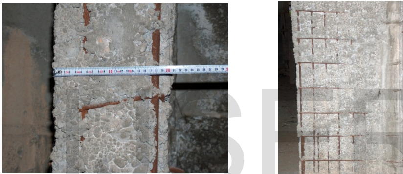
Fig. 15. The concrete cover on the deformed bars is thin
