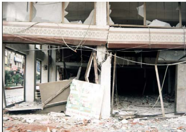
Fig. 10. Shear failure at column Top [24]
