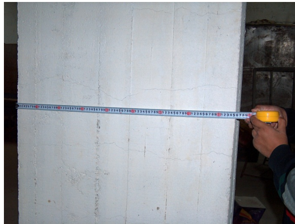
Fig. 21. Cracks caused by creep
