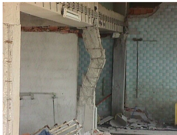
Fig. 4. Typical column failure
