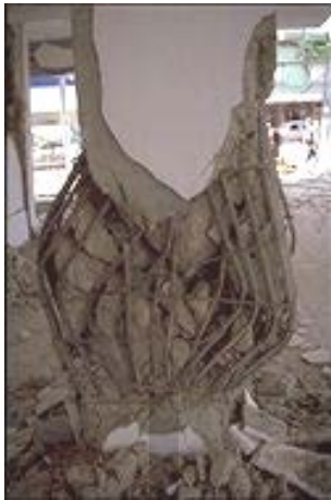
Fig. 18. Failure of short lap splices in moment-column frame
