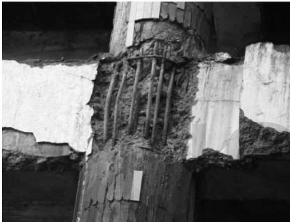
Fig. 9a. The Lack of Shear reinforcement failure of the column [22]
