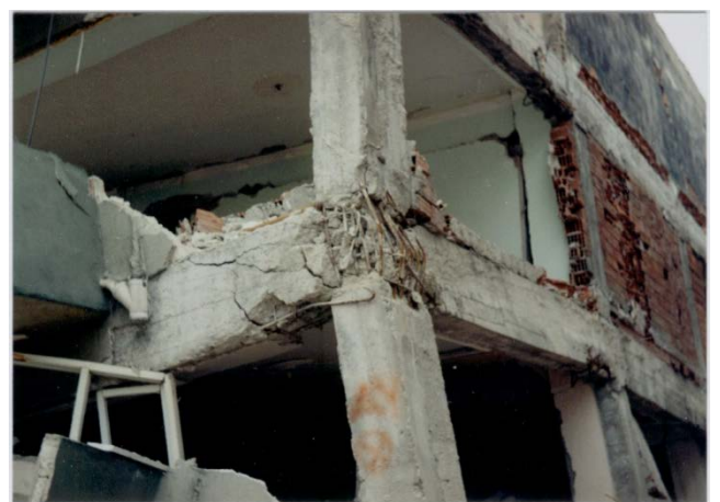
Fig. 23b. Figure Damaged column-beam joint
