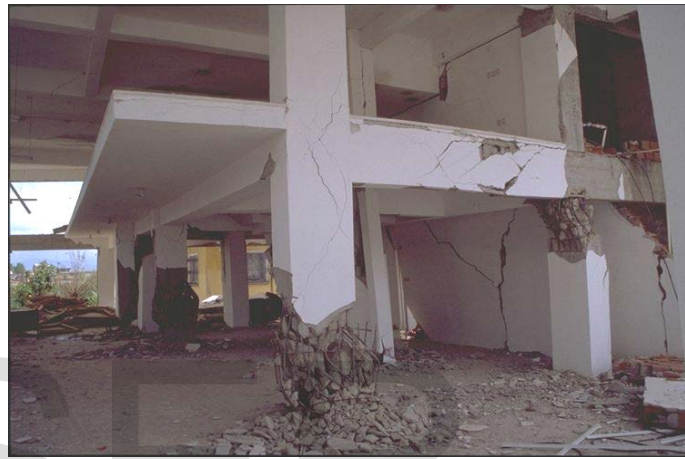
Fig. 19. Short columns failed
