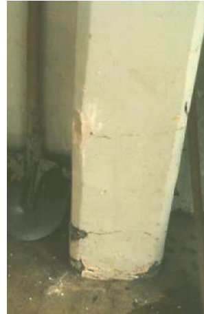
Fig. 2b. Bending cracks witnessed in a coffee-processing factory in Izmit
