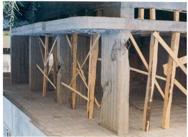
Fig. 8.A damaged column by shear effect
