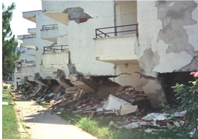
Fig. 5. Strong beam-weak column failure example
