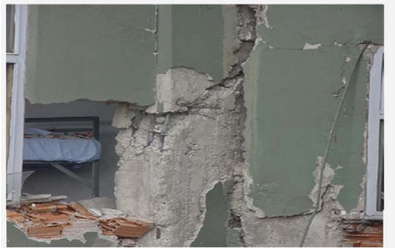
Fig.11. Shear failure of column [26]
