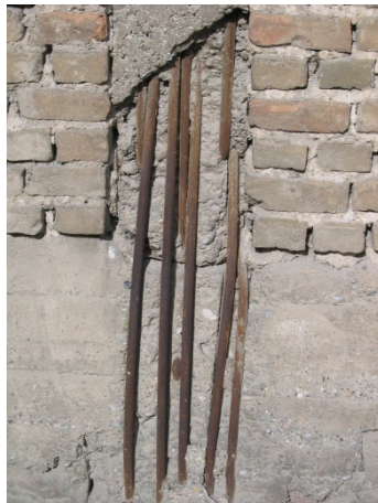
Fig. 14. Longitudinal reinforcement of a column is not closely spaced (450-600 mm)
